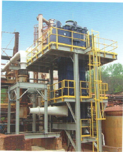
Rockwood Pigments, USA: WESPs save energy with aqueous flushing of collectors instead of mechanical rappers
